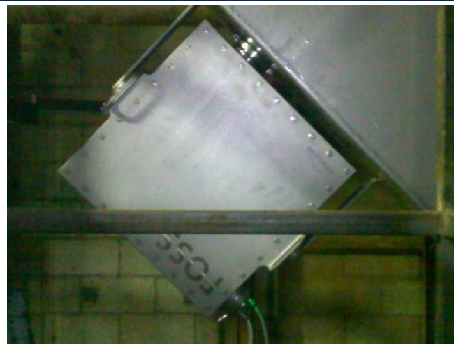
ProFoss installed on open chute
