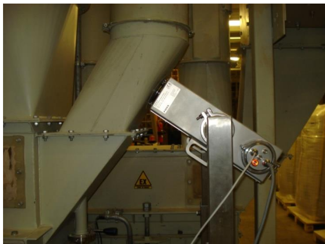
ProFoss installed after mixer
