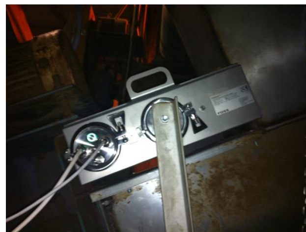
ProFoss installed chute feeding conveyor
