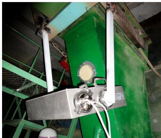
ProFoss installed on chute
